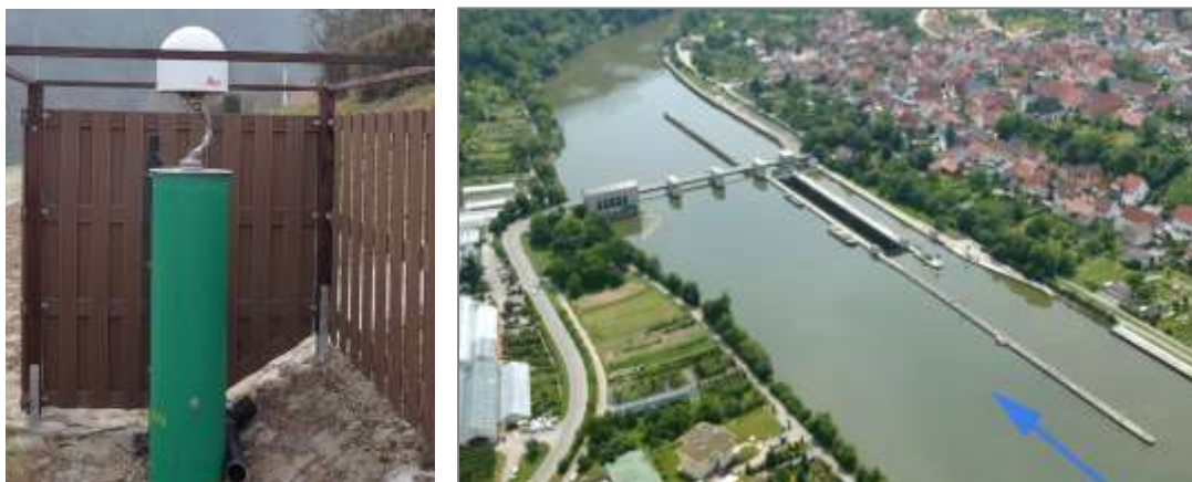
Figure 6: One of the two permanent stations at the Hessigheim water gate for purposes of monitoring
