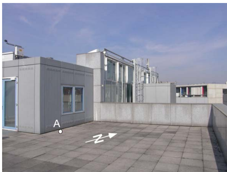
Fig. 3: Antenna location A on roof of TUG building during experiment.
