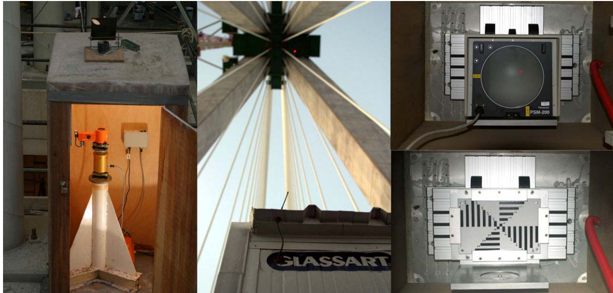
Figure 16: Laser device for measuring pylon base horizontal displacements
